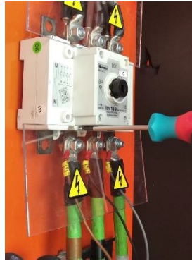
Figure 20: Electrical safety panel
